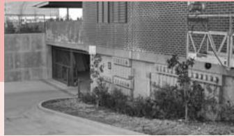
The electrical bank is located on the side of the building, near the lower level entrance of the parking structure. Service access is preserved while the appearance of the electrical bank is minimized.
