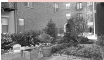
The transformer equipment pictured in this photo (in center of photo behind tall shrubbery) is located within an interior courtyard and screened with landscaping
