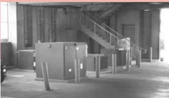
Transformer and switchgear structures are located on the first floor of the parking structure instead of being placed in highly visible locations within the development center.
